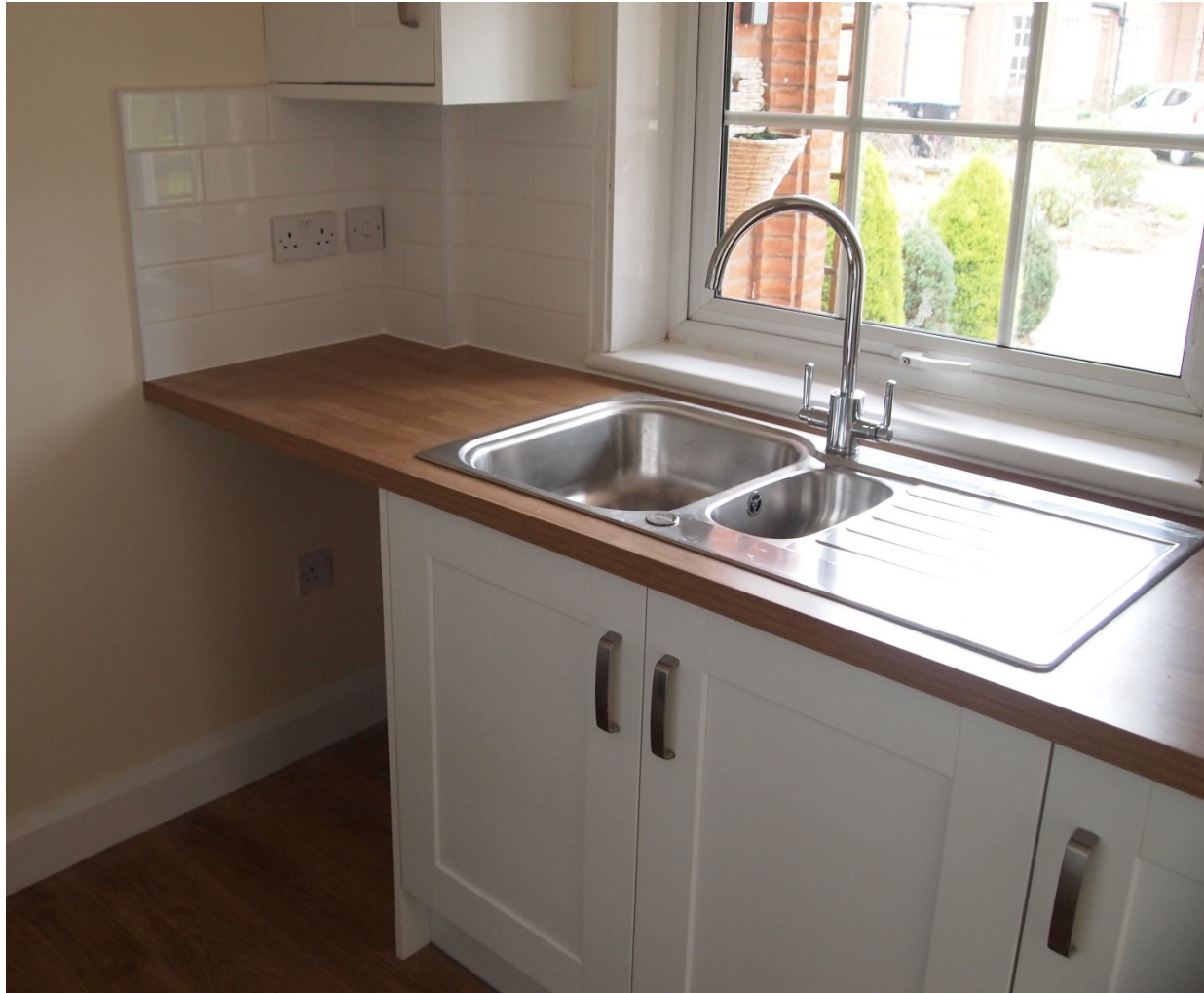
A refitted kitchen with an electric oven and hob
